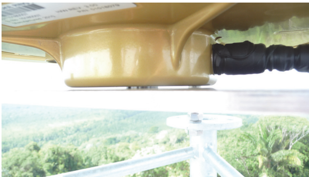
Figure 6: Left) Example of antenna deficiency (AR25)
